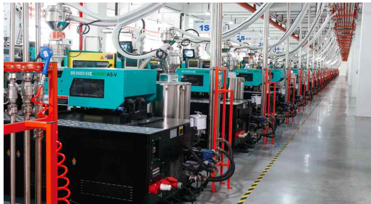
▶ 中央集中自动供料系统 Central centralized automatic feeding system
